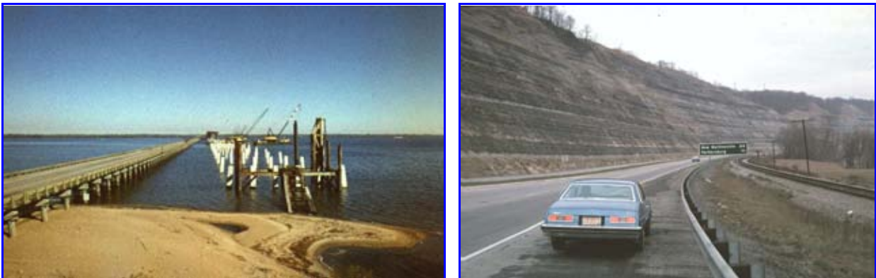
Figure 2-1: New Highway Construction: (a) Pile Bent Bridge in NC and (b) Cut Slope in VA.
