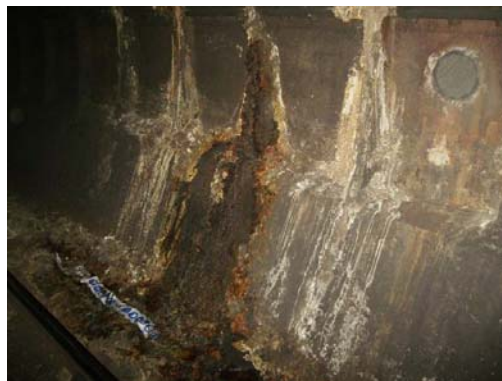
Acid attack by bacteria action on cast iron tunnel lining?
